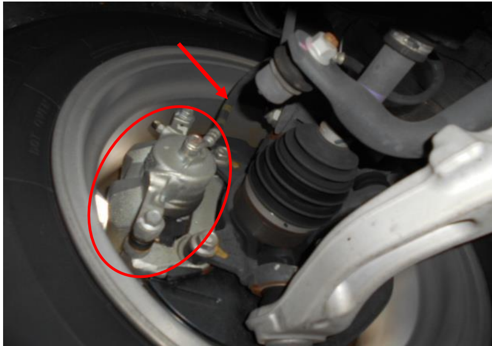
Photo 20 shows the brake hose/pipe (arrowed) at the front right wheel of the Motor Car. I did not observe any leakage of brake fluid at the time of my inspection of the Motor Car. Static tests of the Motor Car's braking system had indicated that there was no internal leakage of pressure/vacuum.
