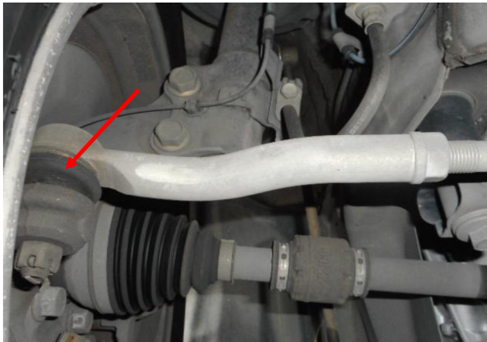
Photo 26 shows the various undercarriage components at the front left wheel of the Motor Taxi, in particular the steering tie rod end (arrowed). The various undercarriage components of the Motor Taxi were all found to be intact without any visible damage. There was also no sign of fluid stain(s) observed on the various undercarriage components.
