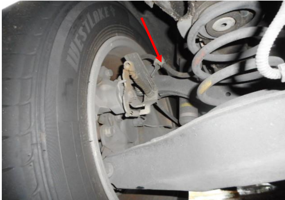
Photo 20 shows the brake hose/pipe (arrowed) at the rear left wheel of the Motor Taxi. No leakage of brake fluid was observed. Visual examination of the various components of the braking system like the drum brake, brake booster, brake pedal etc. had revealed all to be intact and without visible damage.
