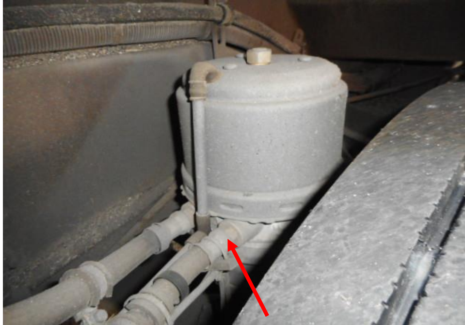
Photo 16 shows the brake pipe (arrowed) at the rear right wheel of the Motor Bus. I did not observe any leakage of brake fluid at the time of my inspection of the Motor Bus. My static tests of the Motor Bus's braking system, along with my visual examination of the various mechanical components in the braking system, had indicated that there was no internal leakage of pressure/vacuum. Hence the braking system of the Motor Bus was likely to be in serviceable condition at the material time of accident.
