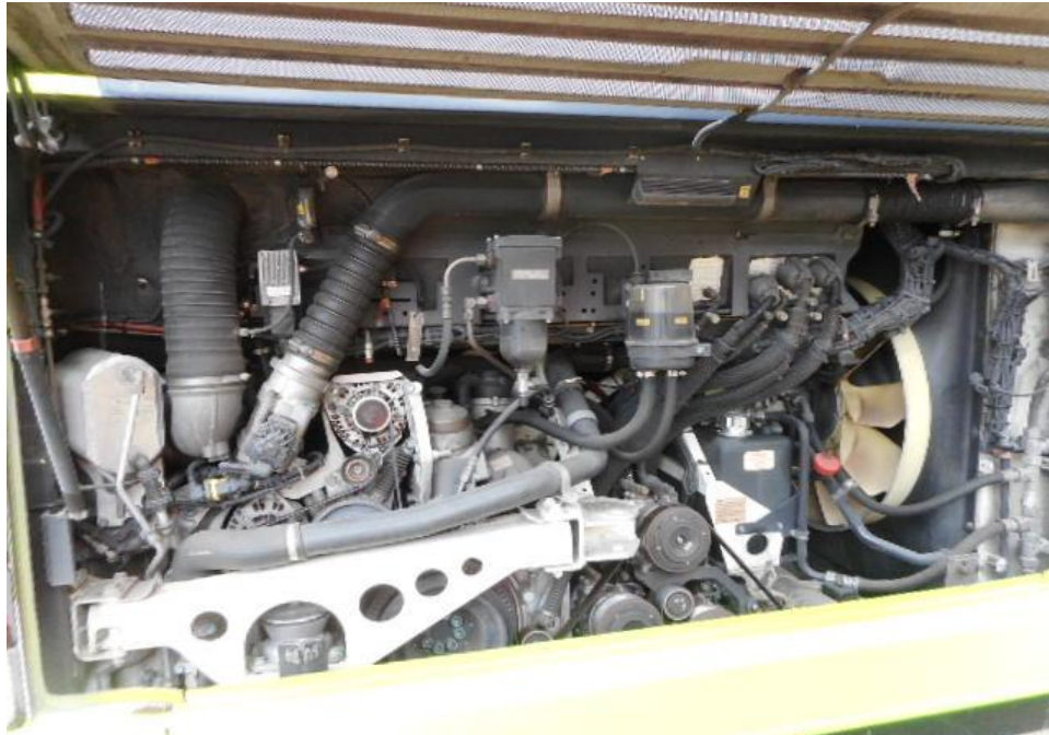
Photo 11 shows a general view of the Motor Bus's engine compartment, which was accessed by lifting the rear of the Motor Bus. The various parts and components inside the engine compartment were unaffected by the accident. There was also no sign(s) or indication(s) of fresh fluid leakage and/or fluid stain within the engine compartment
