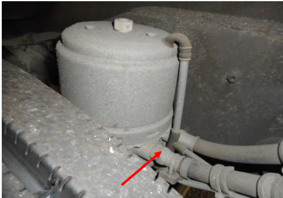
Photo 17 shows the brake pipe (arrowed) at the rear left wheel of the Motor Bus. I did not observe any leakage of brake fluid at the time of my inspection of the Motor Bus. My static tests of the Motor Bus's braking system, along with my visual examination of the various mechanical components in the braking system, had indicated that there was no internal leakage of pressure/vacuum. Hence the braking system of the Motor Bus was likely to be in serviceable condition at the material time of accident.
