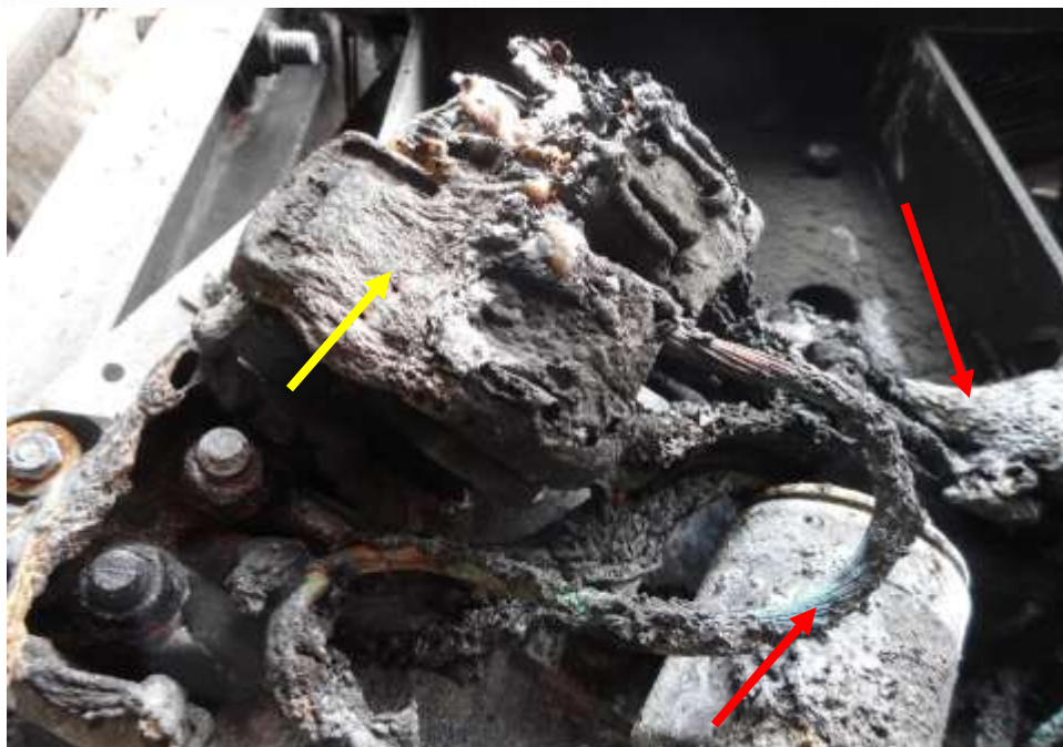
Photo 12 shows close up view of the original wiring harness from the batteries (red arrow) to the electrical components (yellow arrow) was observed with greenish residue on the surface. The presence of greenish residue indicates internal heating of copper wires, a sign of an electrical short circuit occurring. The greenish residue is normally left behind from oxidation as a result of chemical reaction involving the copper wires.
