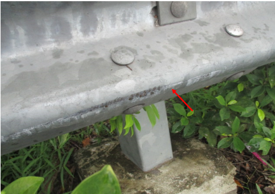
Photo 5 shows a close up view of the whitish paint graze marks along some of the railings (arrowed).
