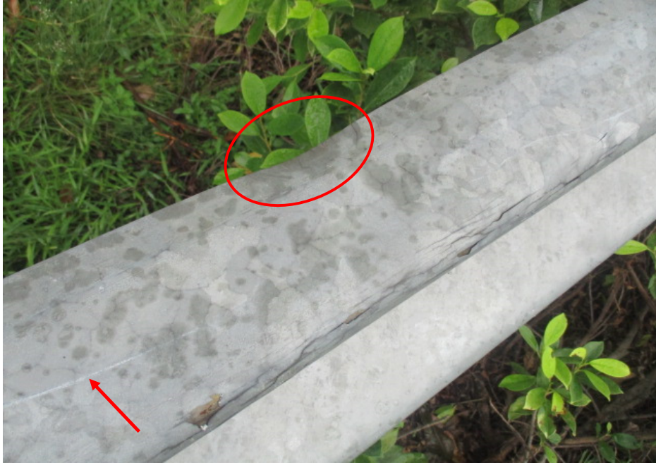
Photo 6 shows a close up view of the whitish paint graze marks along some of the railings (arrowed). A portion of the railings was also found to be dented (circled).
