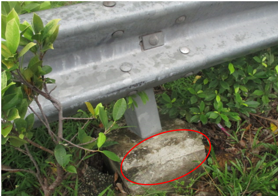
Photo 3 shows a close up view of the minor damage to the base of a railing adjacent to lamp post 635 (circled).
