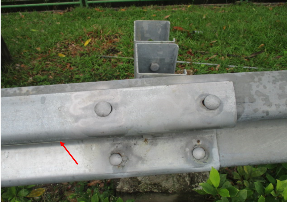
Photo 4 shows upon closer inspection of the railings, we observed whitish paint graze marks along some of the railings (arrowed).
