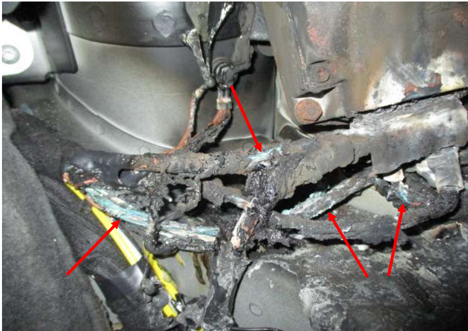
Photo 7 shows the greenish residue (arrowed) that was found on the wirings leading to the burnt connector socket. The presence of greenish residue on the wirings indicate internal heating of copper wires, a sign of an electrical short circuit occurring. The greenish residue is normally left behind from oxidation as a result of chemical reaction involving the copper wires. This physical evidence suggests that the cause of fire to the Insured Vehicle was due to electrical in nature.
