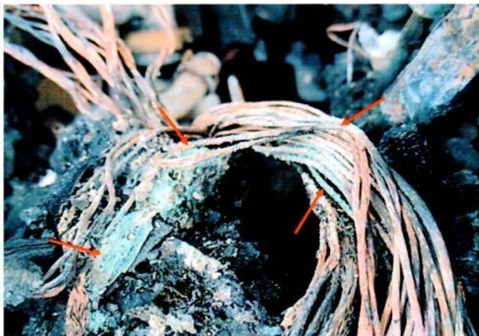
Photo 12 shows a close up view of the greenish residue found on some of the burnt stretches of original factory fitted wirings (arrowed). The presence of such greenish residue suggests occurrence of an electrical short circuit.
