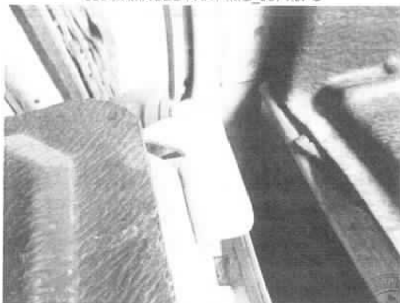
010 DAMAGED PART IMG_0572.JPG
