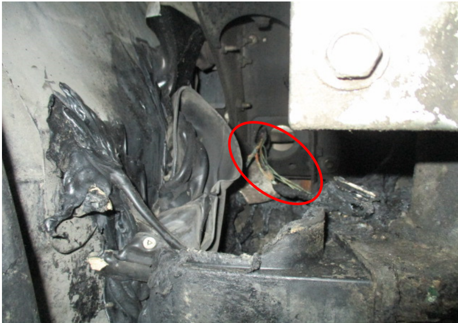
Photo 12 shows a closer view of the greenish residue found on the burnt wirings of the Insured Vehicle's air cleaner assembly (circled). This seems to suggest the occurrence of an electrical short circuit.
