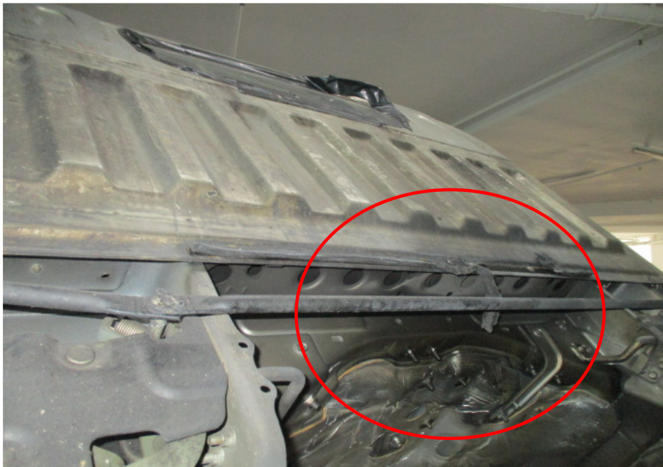
Photo 4 shows the exterior rear portion of the cab of the Insured Vehicle at the time of our inspection. The fire damage to the Insured Vehicle was confined to its centre portion (circled).
